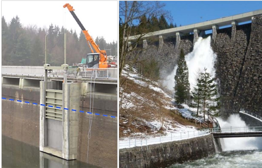
Figure 2: Surface outlet structure. Left: Vertically movable penstock allowing to adjust overflow level (blue line: flood control fill level); right: functional test at approximate maximum outflow capacity of the outlet (10 m 3 /s). Photos: LTV
